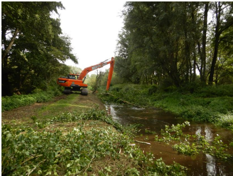
Big machinery placing tree ledges for flow deflection at the Alder Carr reach at West Stow, October 2022
