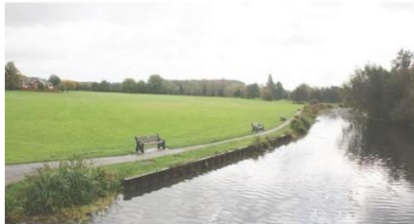
River Lark water levels lowered, creation of riverside access and marginal vegetation
