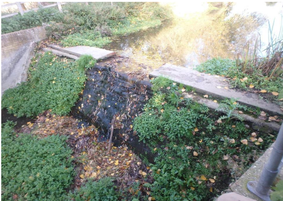
Fig 12. Gas Pool Side weir, notch cut in the weir when the river was last lowered.
