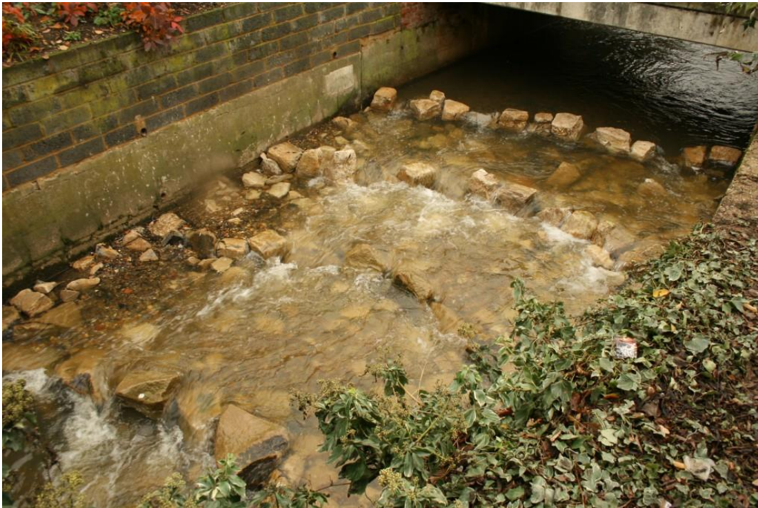
Fig 10. Rock ramp, the bed is lowered and replaced with designed boulder placement, the cross section of the channel is increased improving flood discharge.
