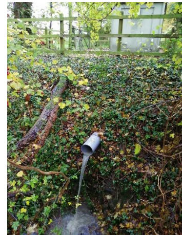
Figure 24: Whepstead pumping station storm overflow occurring in December 2019
