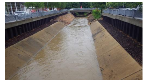
Photo 8: Concrete Lark, St. Saviours Tesco Bury St Edmunds.
